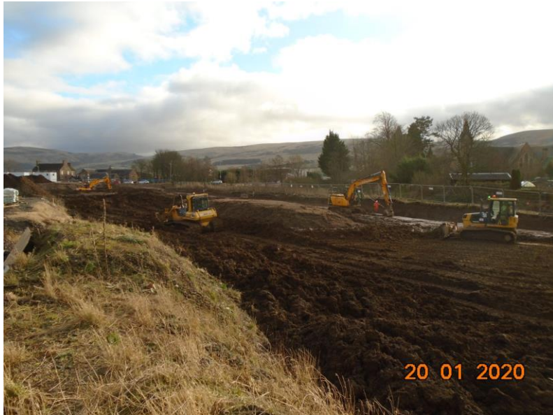
Compensatory Storage Soil Strip
