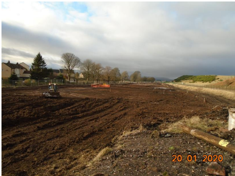
Compensatory Storage Soil Strip
