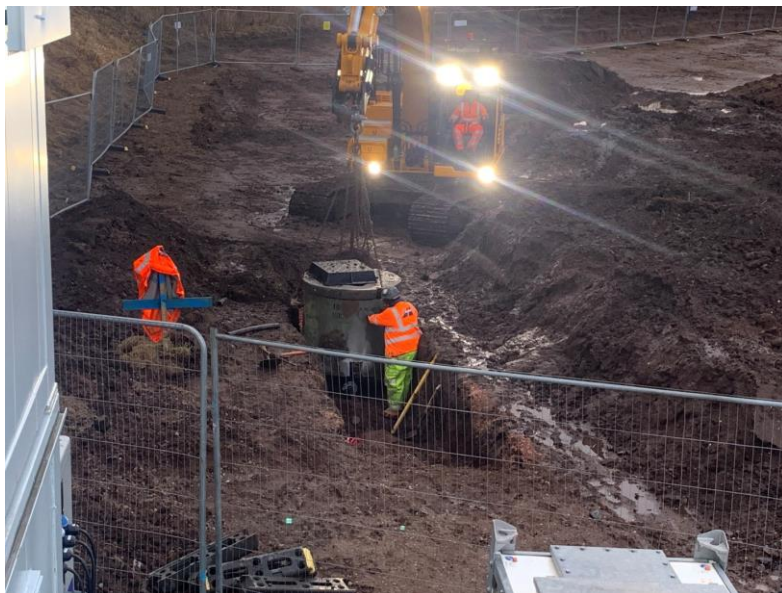
Rising Main Air Valve
