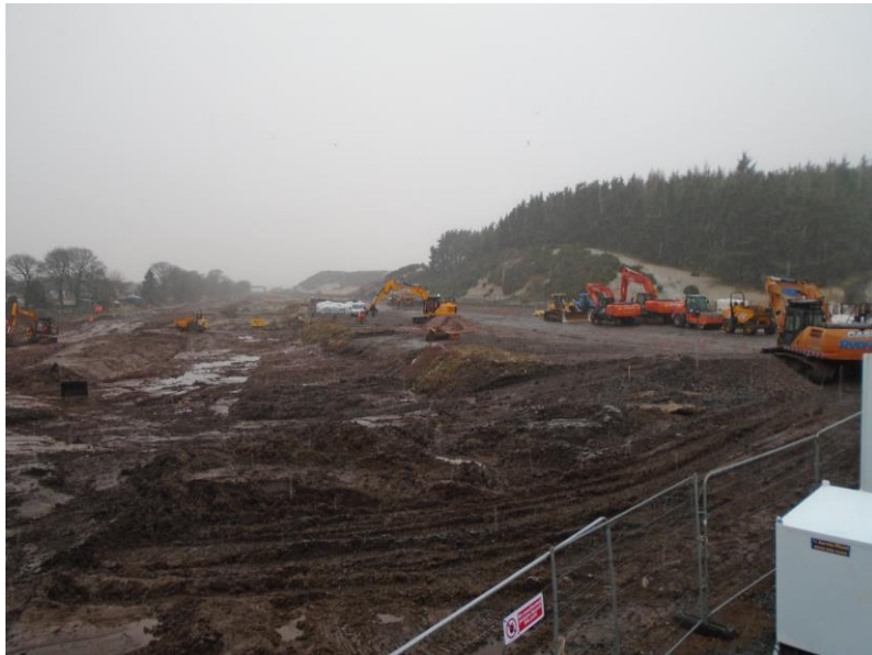
Compensatory Storage Soil Strip
