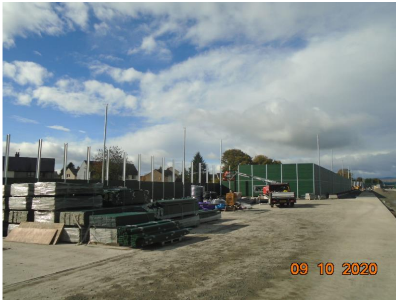
Fencing / Street Lighting
